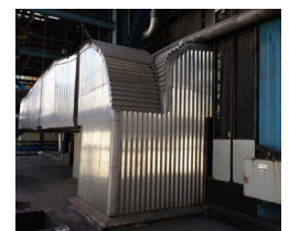
SOFA air duct
