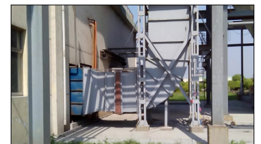
Boiler Flue Gas Duct
