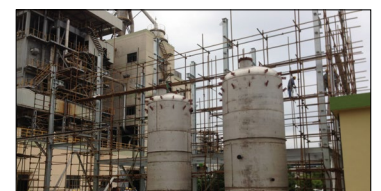
Ammonia Storage Tanks
