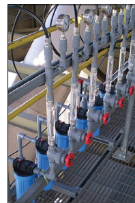
Ammonia Injection Grid
